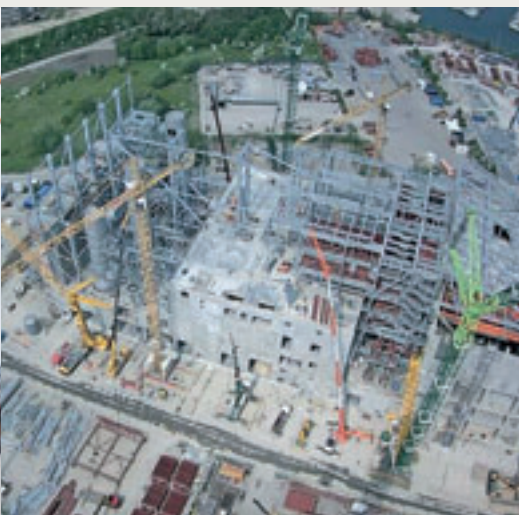
Left: Construction work on the roughly EUR 500 million project is scheduled for completion by 2017. Center: State of progress in May 2015. The steel structure for the 31,000 m 2 roof is gradually taking shape.
