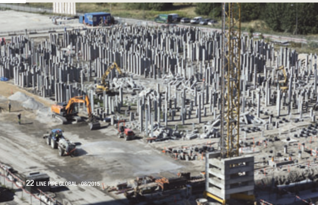
Left: Start of foundation work for the new facility that, with a height of 100 m, is set to be a new Copenhagen landmark.
