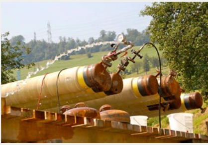
The pipe strings welded together on land were subjected to a pressure test at 7.5 bar.
