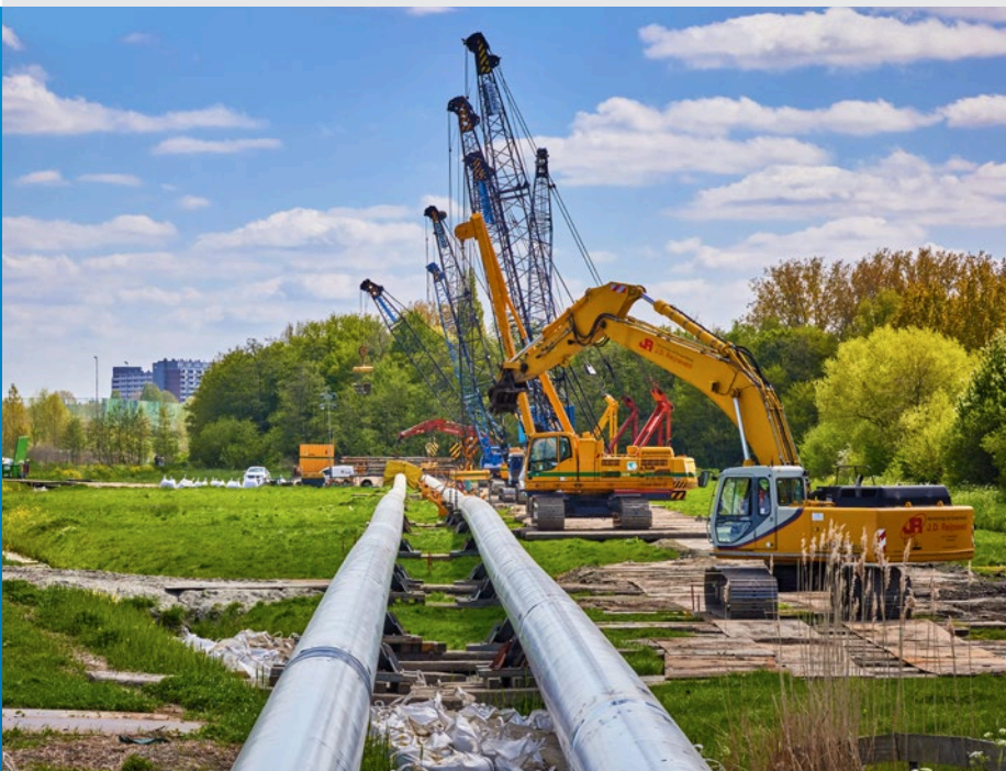
District heating networks are also being expanded in the Netherlands. Mannesmann Line Pipe has supplied 600 tonnes of HFI-welded steel pipes to the WarmtelinQ project. Photo: © WarmtelinQ, Vincent Basler
