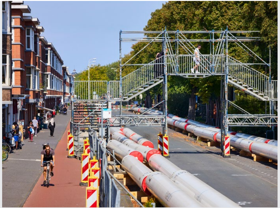
The work on WarmtelinQ is being carried out at up to 30 locations simultaneously. Photo: © WarmtelinQ, Vincent Basler
