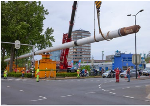
Always great interest in the laying of long pipe strings. Photo: © WarmtelinQ, Vincent Basler
