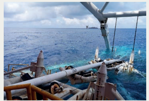
The pipes pressed together to form the pipeline using the Zap-Lok™-method are being laid over a distance of 60 km in the South China Sea.
