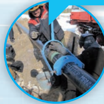
Flowlines – secondary oil production
