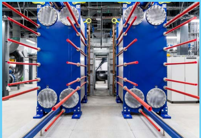
Heat exchangers play an important role in cooling the data center.
