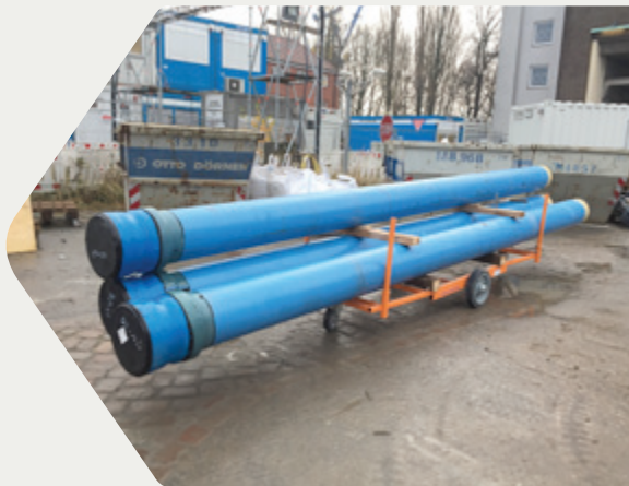
Hand trolleys were used to transport the 6 m long pipe sections to the lifts which took them down to the tunnel tube.
